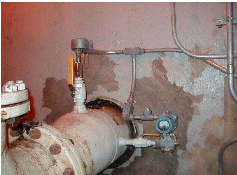
Pressure and Temperature Transmitter on pipe
