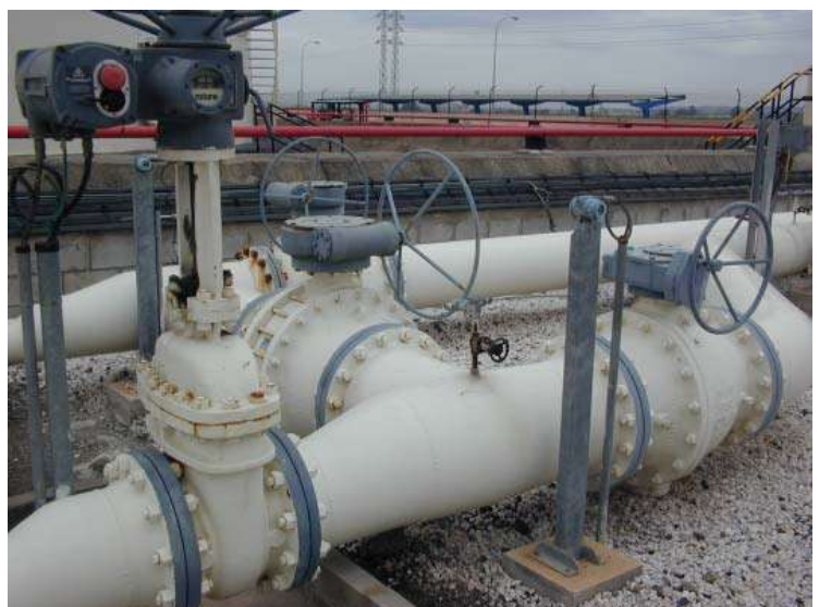
Manual and Motor Operated Valves
