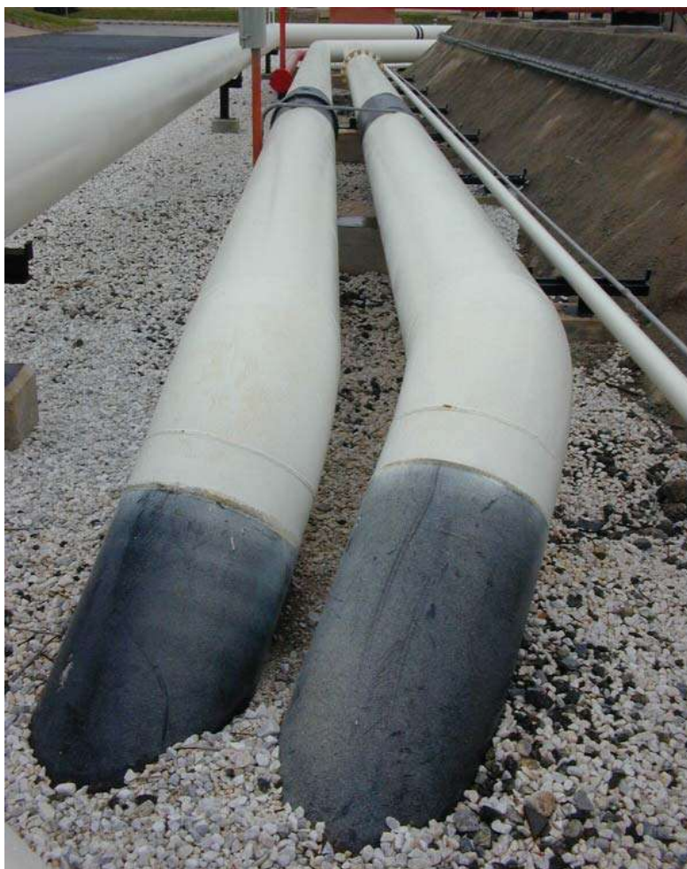
Main hydrant pipes disappearing into the ground
