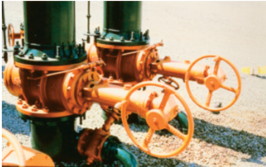
Buried Hydrants Require Regular Pressure Tests
