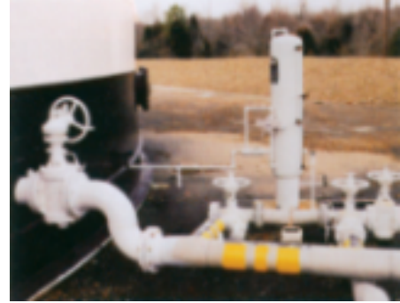
Tank-Side Isolation Maintains Product Integrity
